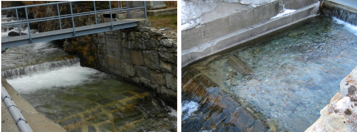
Figure 5 & Figure 6: FOEN gauging station LaRösa, after (left) and before bricking of the riverbed and sealing cracks at the orographic right side (right) (Figure 6 – Andrea Crose / FOEN)
