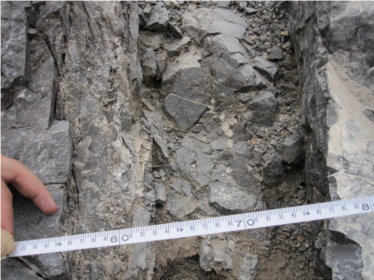
Figure 14: Fractured rock that was clearly caused by the effects of a fault (zone) but did not fit in any of the previous fault rock categories was classified as intensely fractured dolostone.
