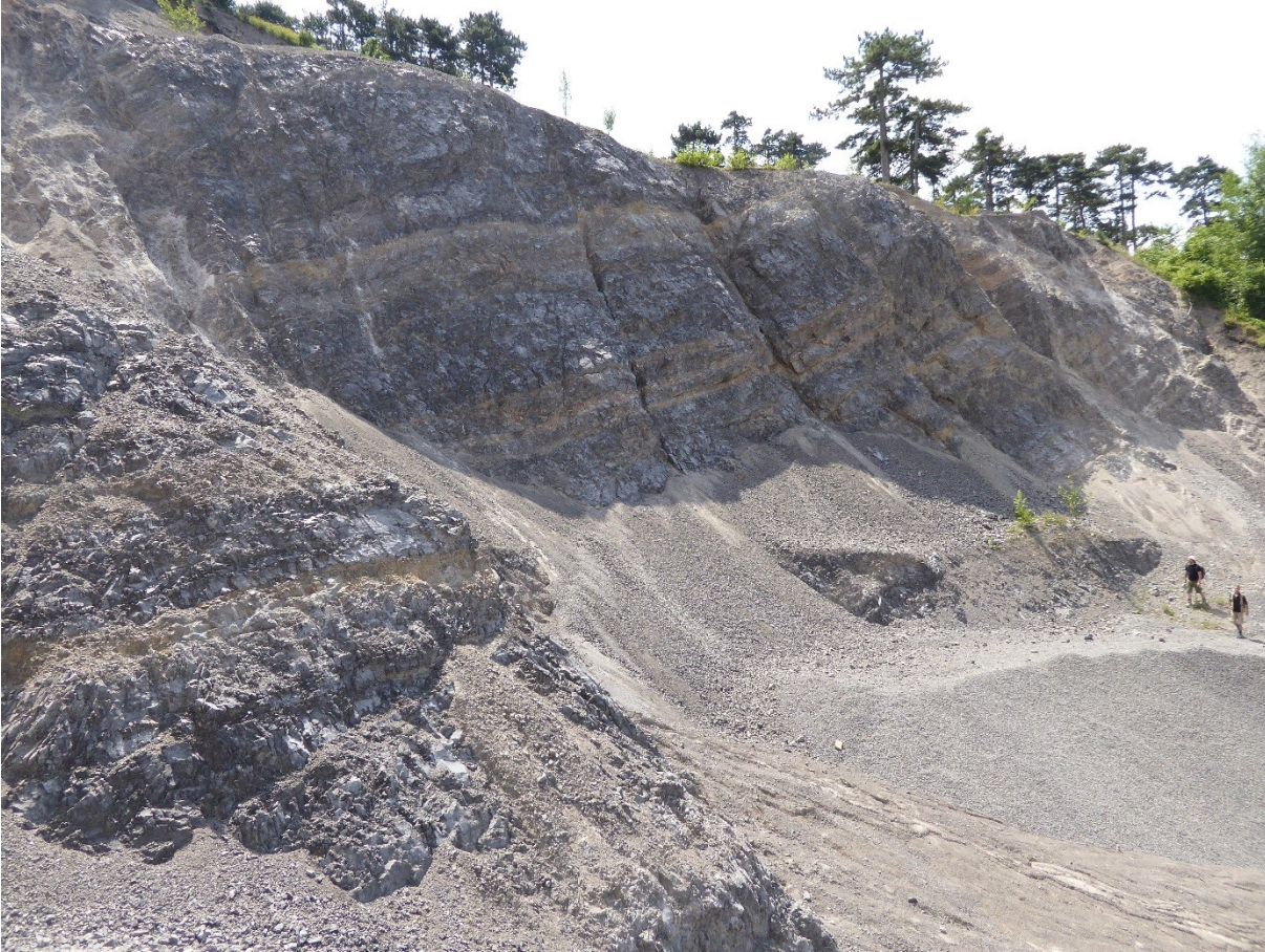
Figure 16: Fracture density varying between individual dolostone beds as visible on the rocks in the foreground. View towards SW.
