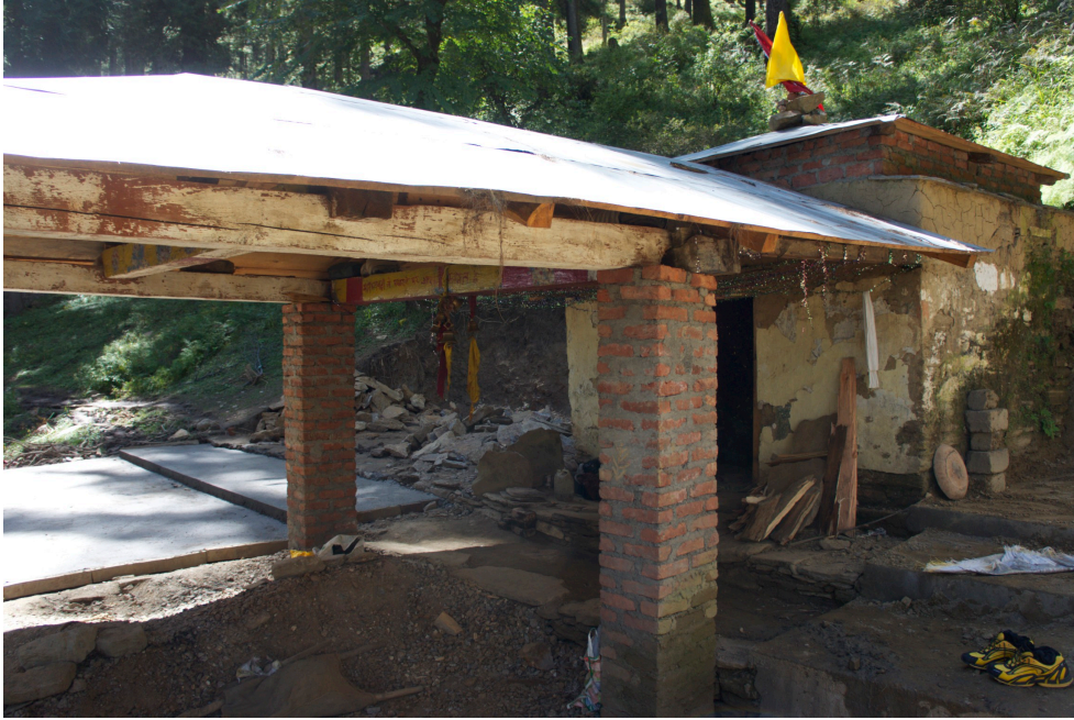
Figure 2.10: The Bhaviṣya Badrī temple under renovation at the time of my visit.
