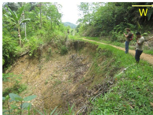
Figure 140: Landslide sliding direction NE
