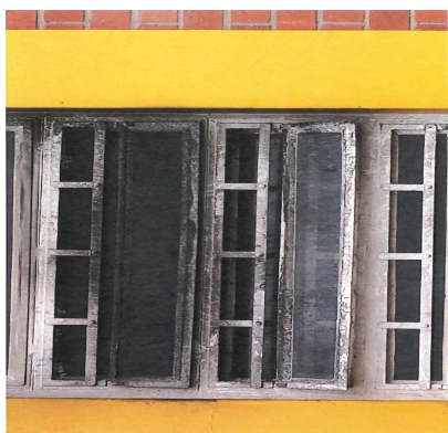
Fig. 14: Soot on cell window after suicide attempt
