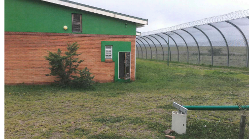
Some of the damage allegedly done by the boys during the 2015 staff strike.
