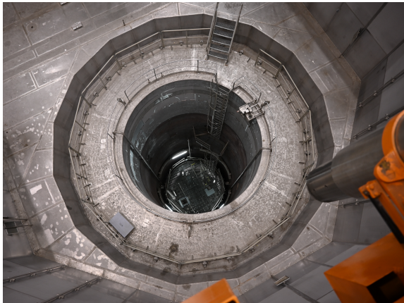
Figure 13: View into the reactor
