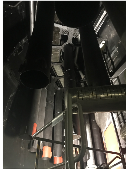
Figure 19: Tubes in the pressure suppression chamber
