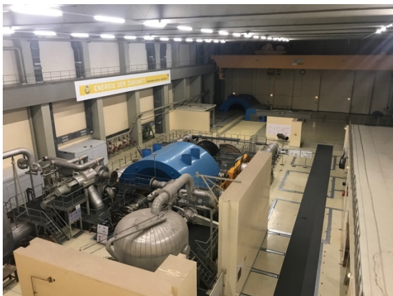
Figure 17: Striking view into the turbine hall
