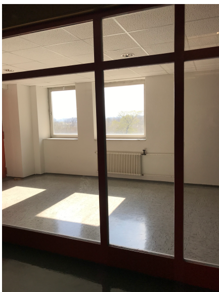
Figure 35: Windows in the control room
