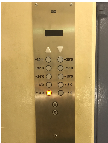
Figure 8: Elevator control panel
