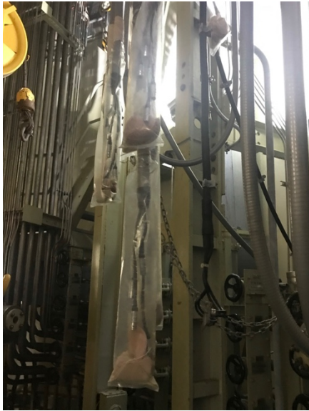
Figure 26: Wrapped-up cable ends
