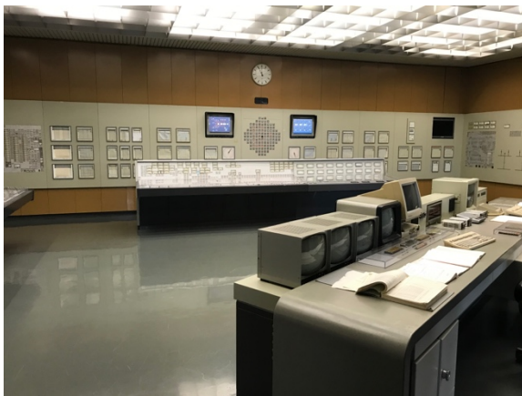
Figure 31: The control room
