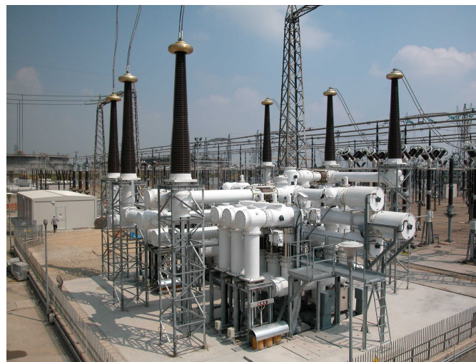
Figure 1.4: \text{SF}_6 gas circuit breakers in a 420 kV switchyard (Dingy 2007).
