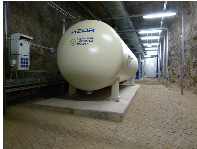
Figure 1.5: SF 6 storage tank at the university of Dresden (Yeti-Hunter 2018).
